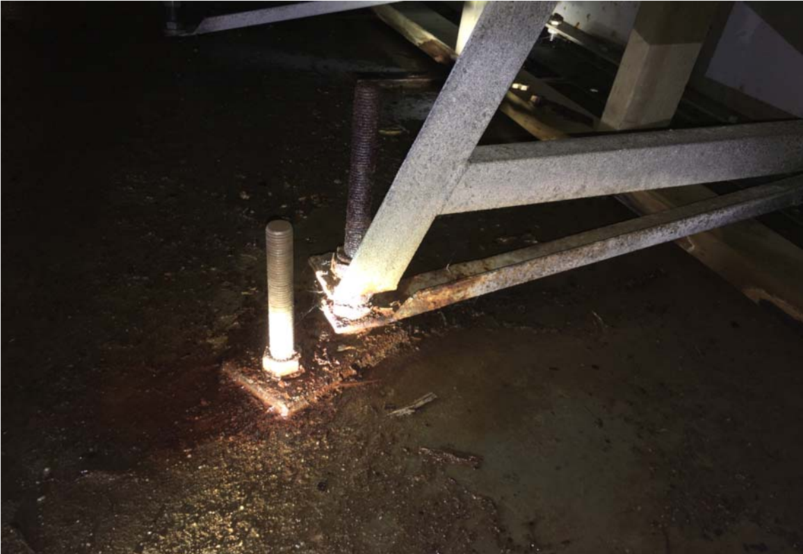
Figure 8: Photos showing anchor bolts corrosion & base plates in 3 different locations.
