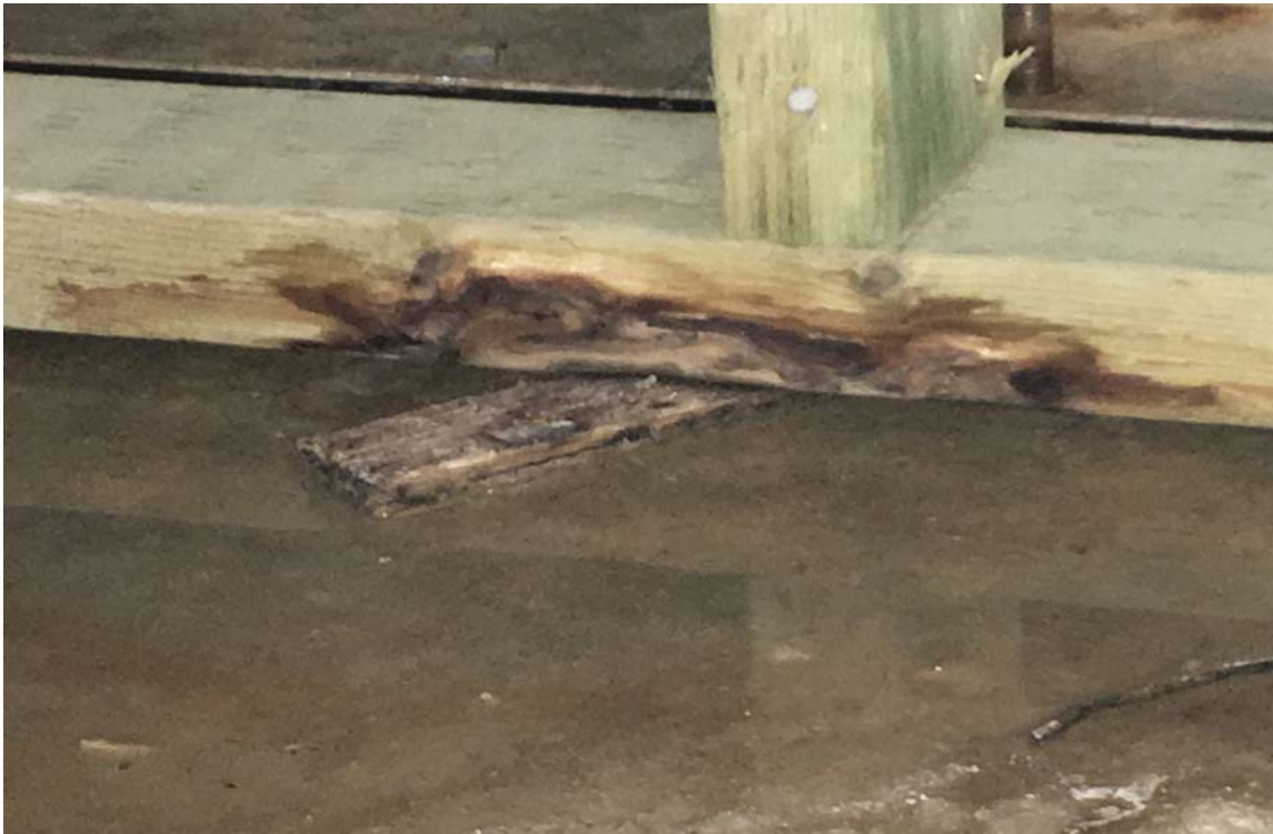
Figure 9: Photos showing bearing wall deterioration of wooden sill plates including log screws corrosion in all areas under water ponding and constant moisture.
