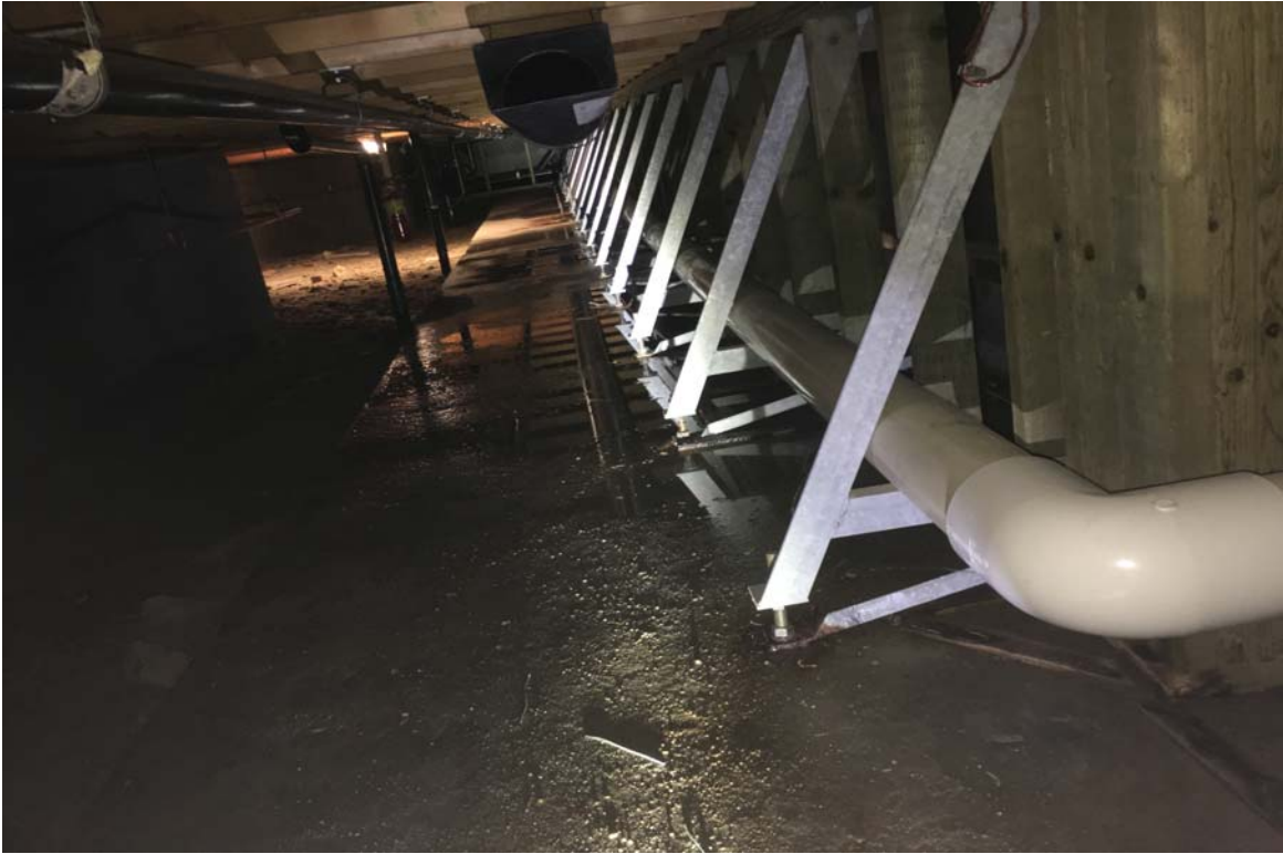
Figure 6: Photos showing water ponding and wetness of the pool concrete slab towards and parallel to Gridline 6.
