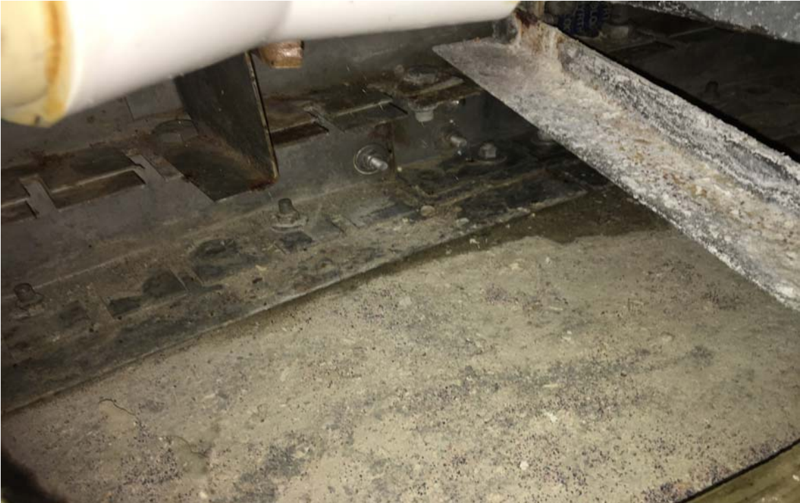
Figure 3: Photos showing water ponding and wetness of the pool concrete slab towards and parallel to Gridline B.
