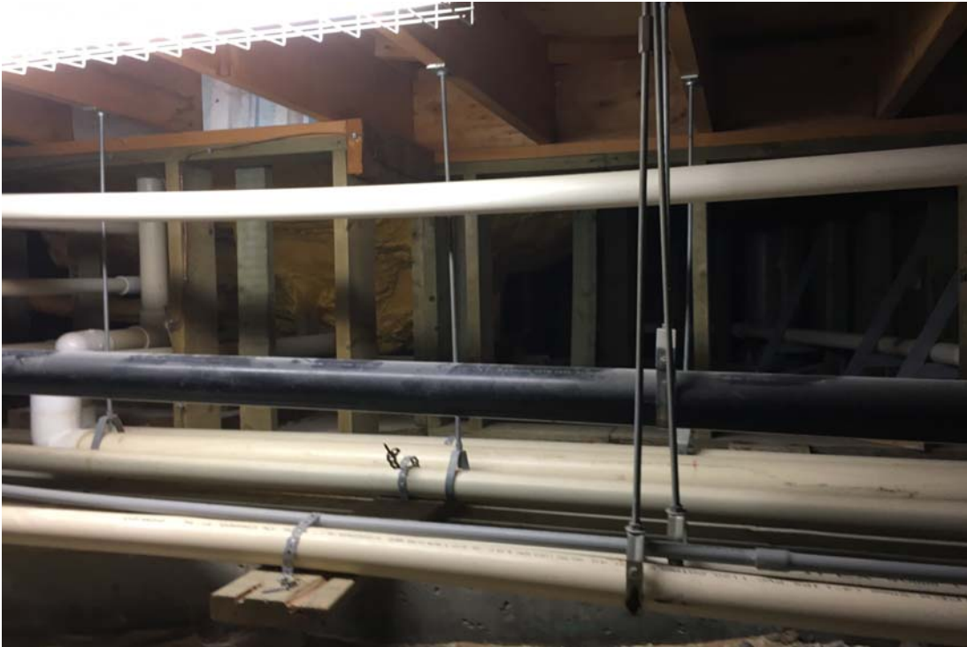
Figure 2: Photos showing buttress support for the whirlpool at crawl space in between Gridline 4 and 5.
