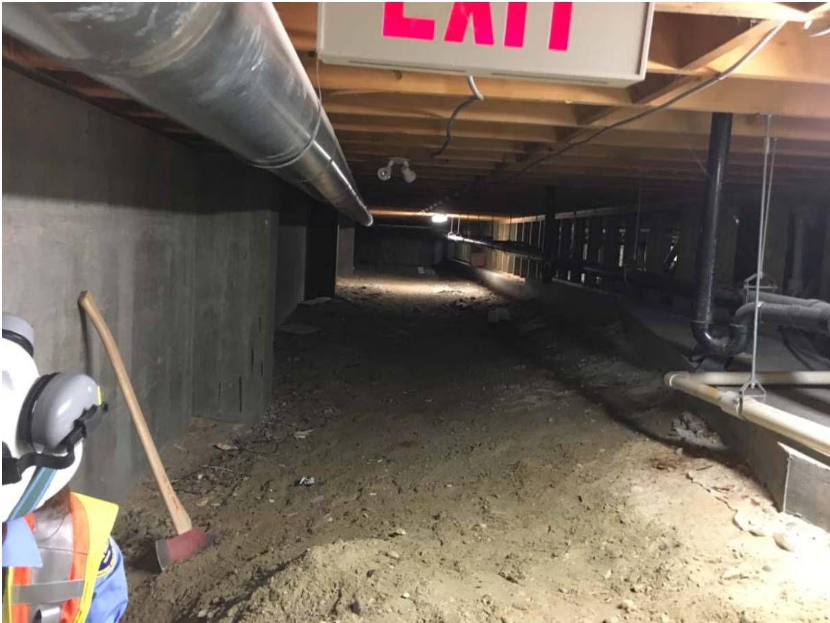
Figure 1: Photos showing existing concrete foundation wall along Gridline B and crawl space access to the swimming pool buttress support and concrete base pad.
