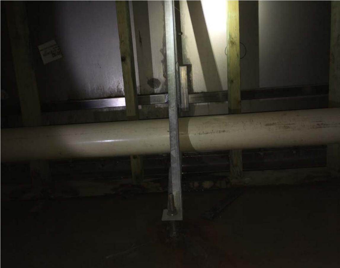
Figure 7: Photos showing water leaking from the wall of the pool parallel to Gridline 6.
