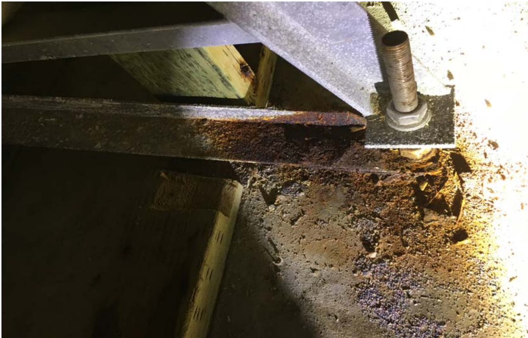
Figure 10: Photos showing corroded horizontal brace at the bottom and base plates in almost 80% of the buttress supporting the swimming pool structure.
