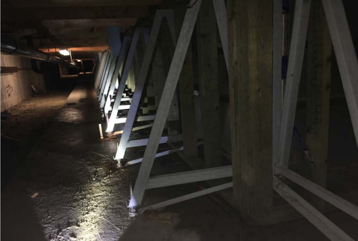
Figure 5: Photos showing water ponding and wetness of the pool concrete slab towards and parallel to Gridline A.
