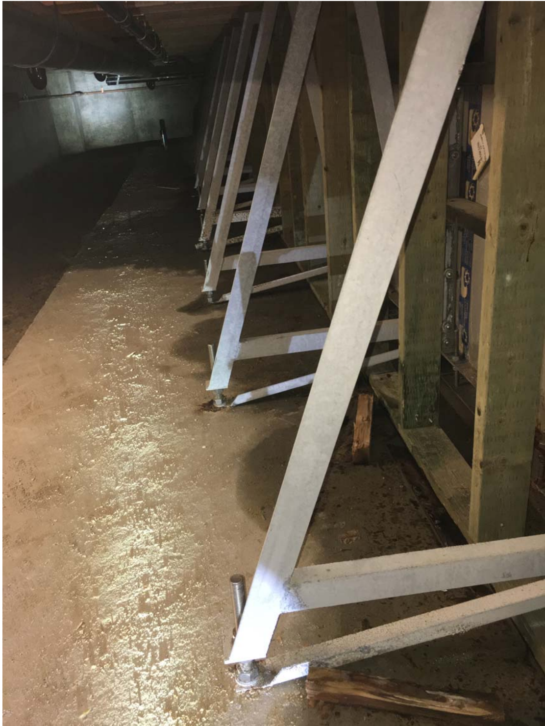
Figure 4: Photos showing water ponding and wetness of the pool concrete slab towards and parallel to Gridline 1.
