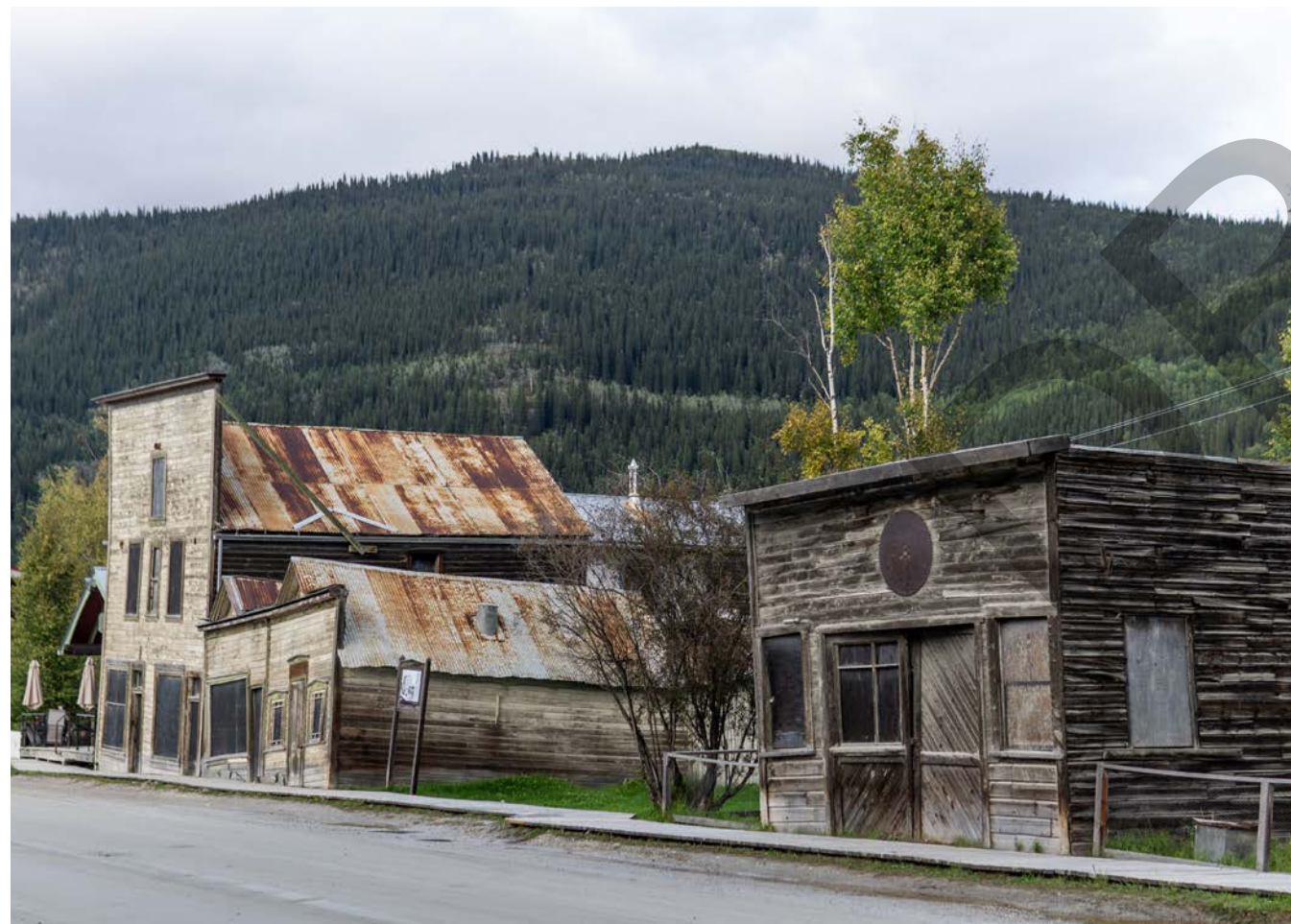
Figure 5: Third Avenue Hotel Complex, colloquially known as the “kissing buildings” as the building is slanting due to permafrost degradation and has been stabilized by Parks Canada
